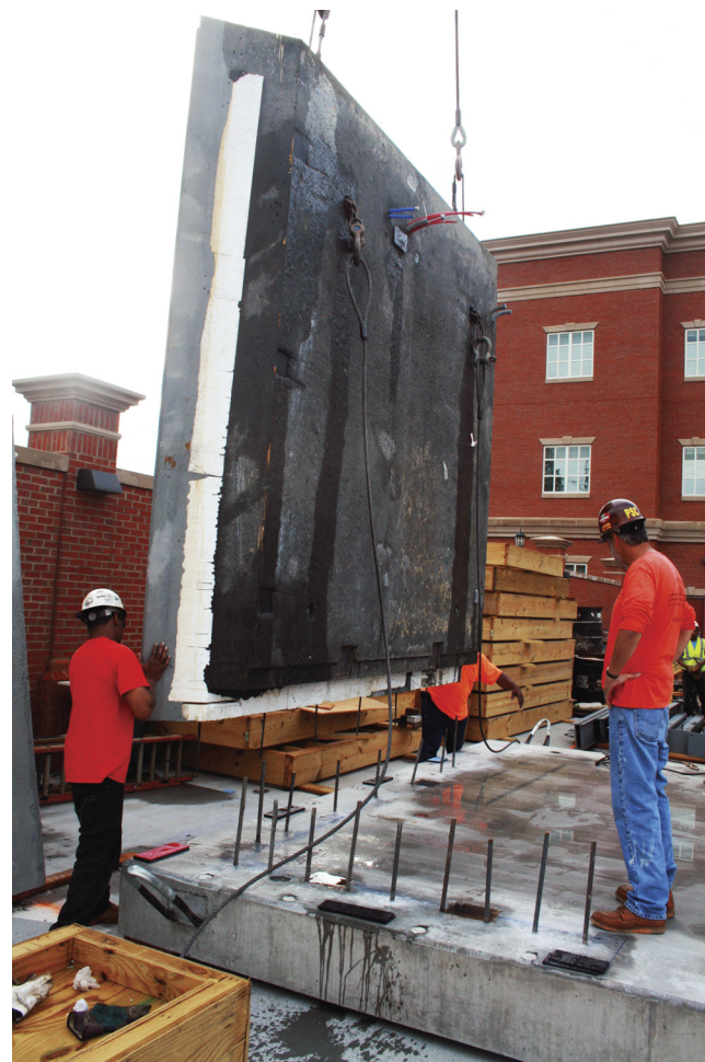
Fig. 1. Continuously insulated precast wall panel being installed as part of a net zero energy project (image by Clarke Snell)
